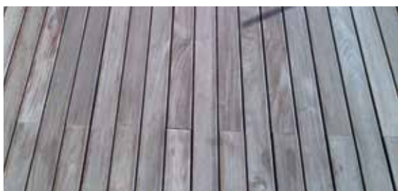
wood terrace after UV weathering without protection
